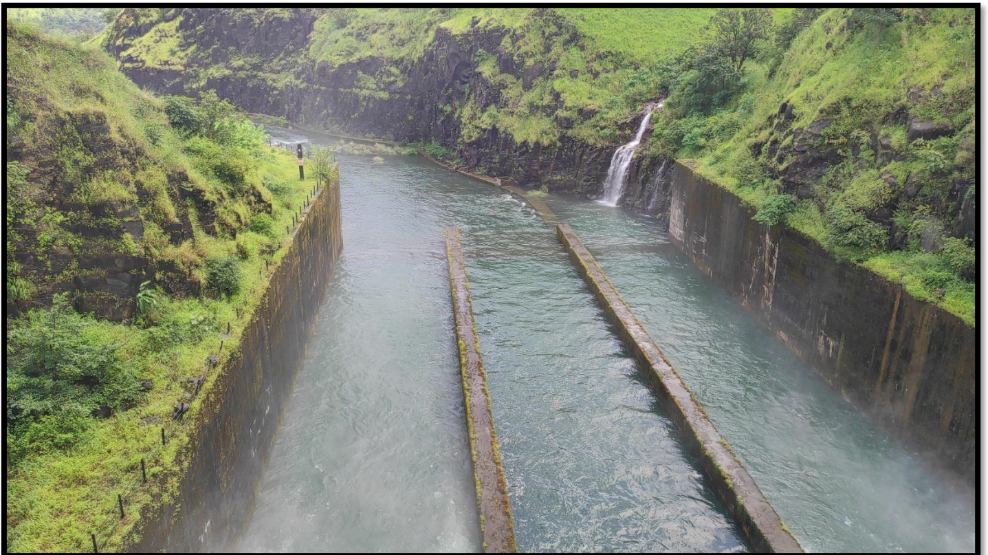
Fig. 7: Water released from Spillway is flowing further through channel to meet river with energy dissipation mechanism further in downstream side through occurrence of Hydraulic jump
