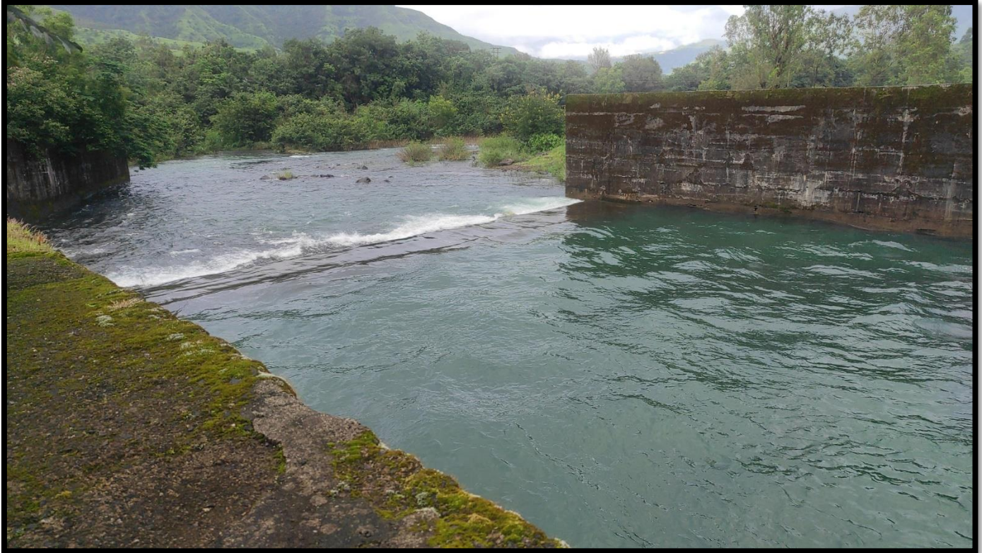
Fig. 30: Water released from spillway comes down along the channel from higher elevation to lower level upto river course. This is end of spillway channel. [ Flip Buckets: If a dam has a steep spillway or chute, a flip bucket at the end of the spillway may be used. The flip bucket causes the water to leap into the air, dissipating energy before the water lands in a plunge pool or stilling basin below.]
