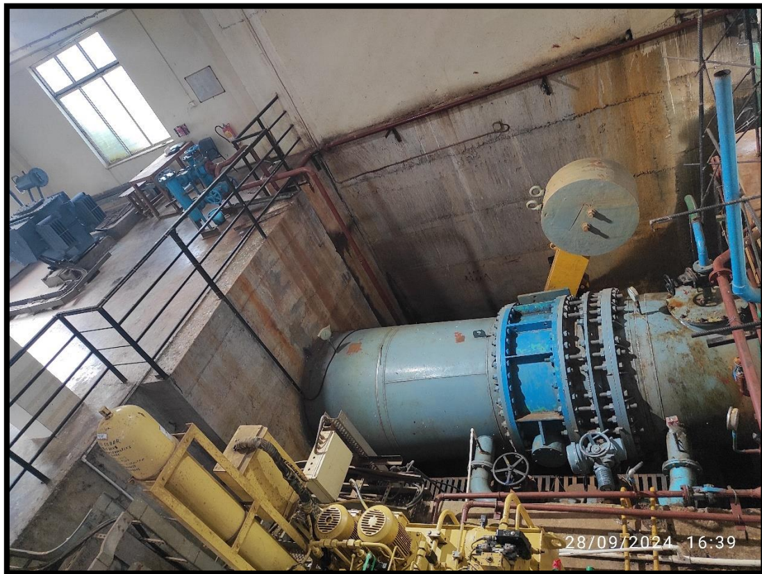
Fig. 21: Penstocks (pipe seen in photo) bringing water under huge pressure head (potential to Kinetic Energy) in the hydroelectric power plant at the toe of Dam. Further this pressure and KE is converted into Mechanical energy after impacting on Impellers of reaction turbine and as shaft starts rotating further Electricity is generated in generator and water comes outside through draft tube at lower level.
