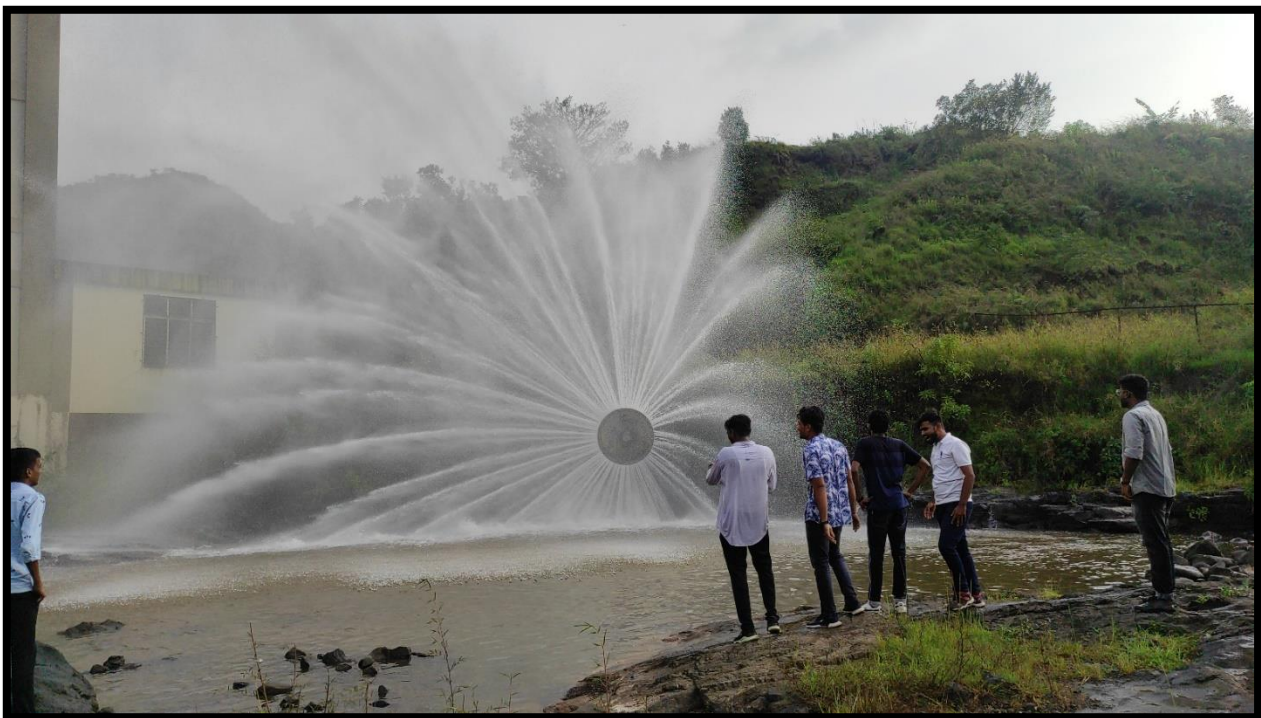
Fig. 26: Butterfly valve is used on Penstock before water enters into power plant (It's like Y distribution system). It serves many functions like regulating water flow, managing water distribution, controlling pressure, and ensuring the dam's safety, Shut-off Function, water diversion. As power plant plant working with full load this time, so missed demonstration of butterfly valve this time.
